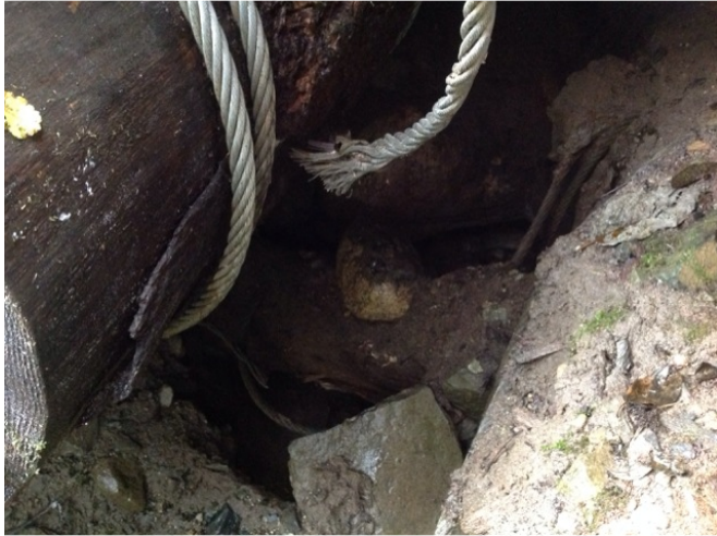
right bank downstream hole under sill
